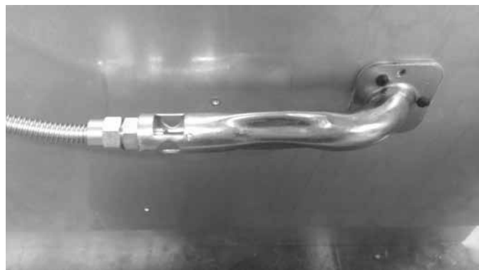
Fig 9.2 Air Shutter Removed Propane Gas
