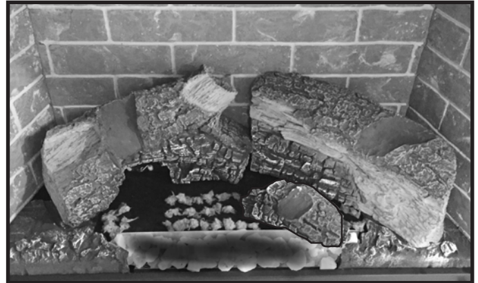
Figure 6 Burner Log Installed
