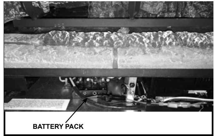
Figure 6.3 Battery Pack Installed
