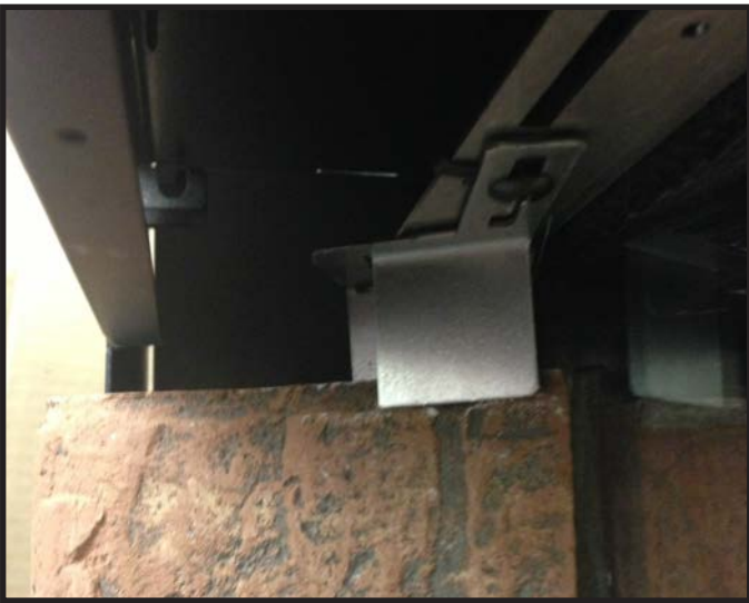
Figure 11.27 Side Refractory Brackets
